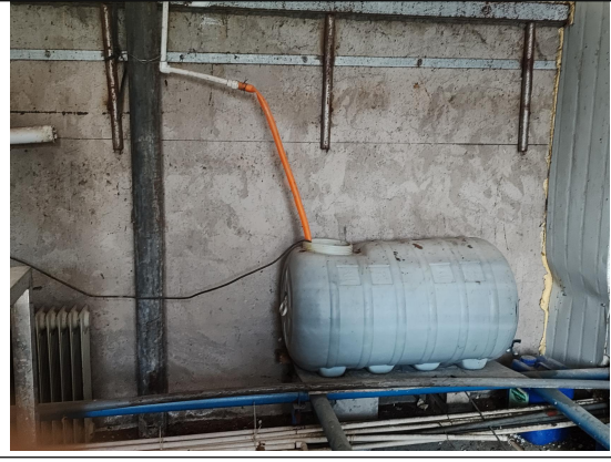
除臭剂加药罐
